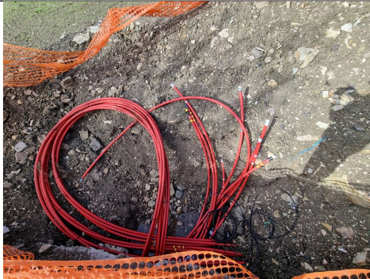
MV line joints
