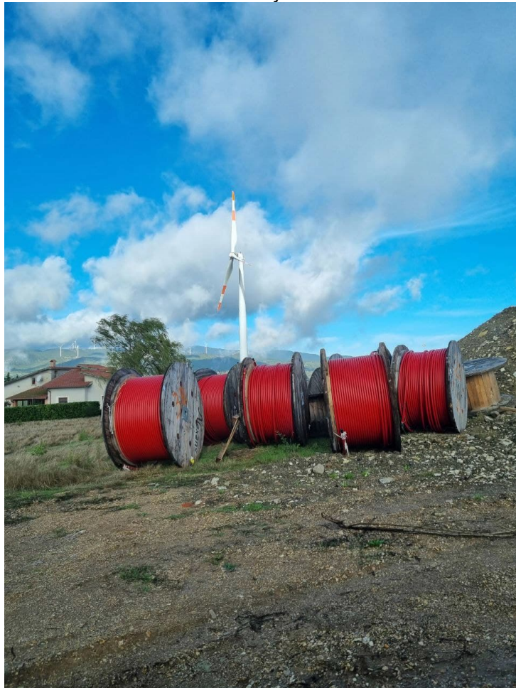
Cable coils stored near the substation for the completion of the remaining 700 meters of the MV cable line of the 3 turbines plot.
