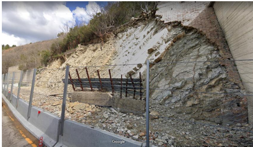
Figure 5-2 - Landslide on SS 90
